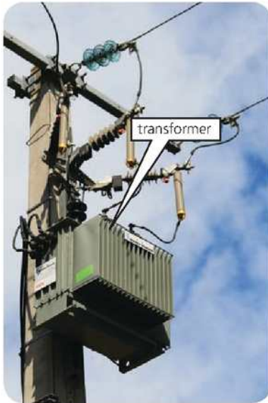
▲ A transformer connected to local power lines
